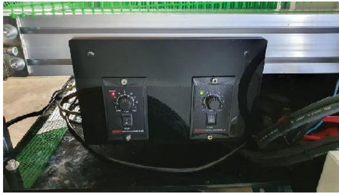
Figure 5 Conveyor Control Box
